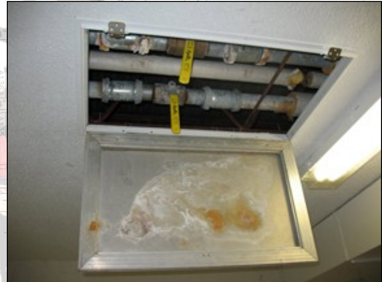
The Boy's Showers are Shut Off Nightly with these Valves to Save Water Since the Shower Faucets Leak Uncontrollably
