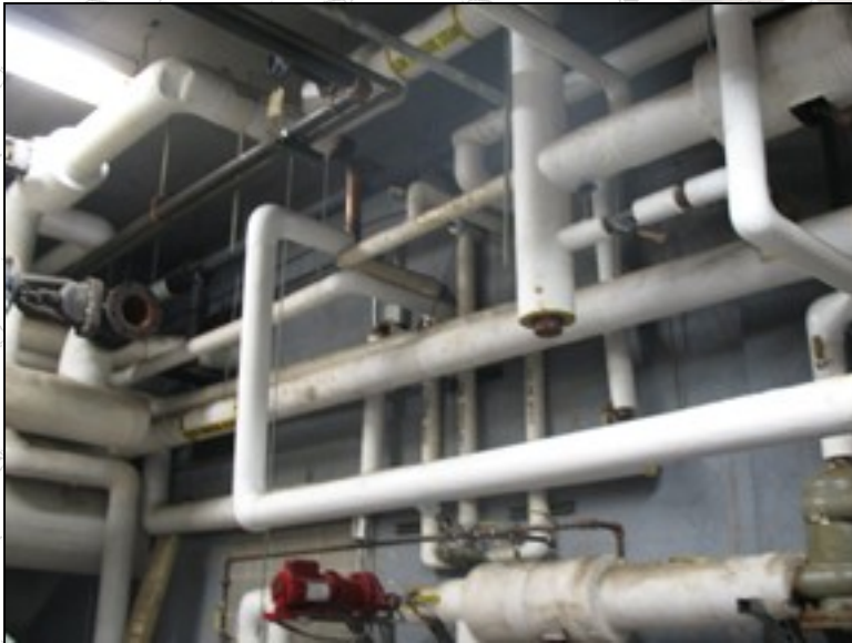
Maze of Abandon Piping in the High School Boiler Room
